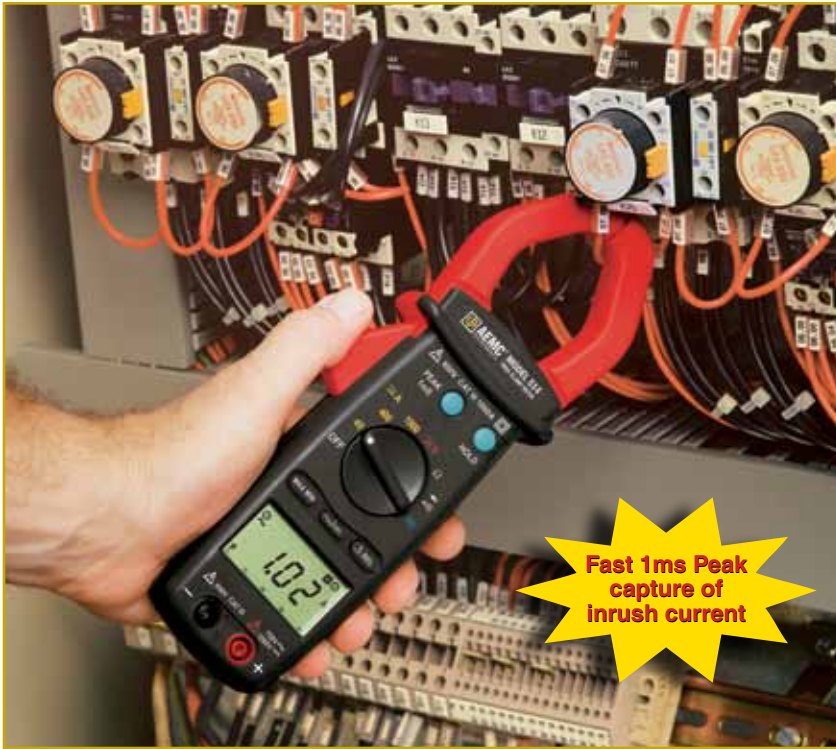
Model 514 measuring primary current on a machine control system.
